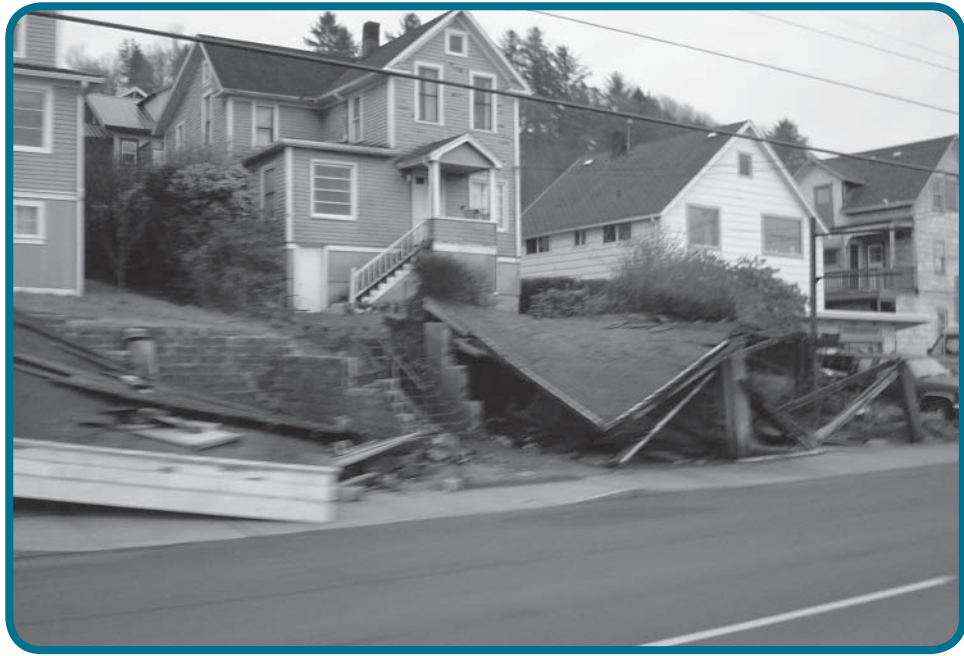
Damage from windstorm Coastal Gale
